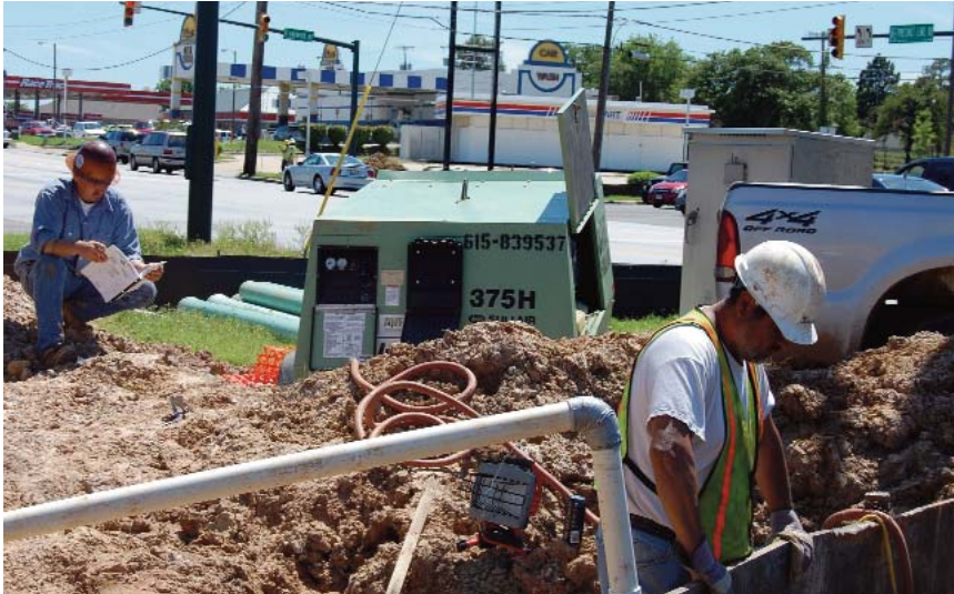
Workers continue to relocate water mains in preparation for the road widening.
